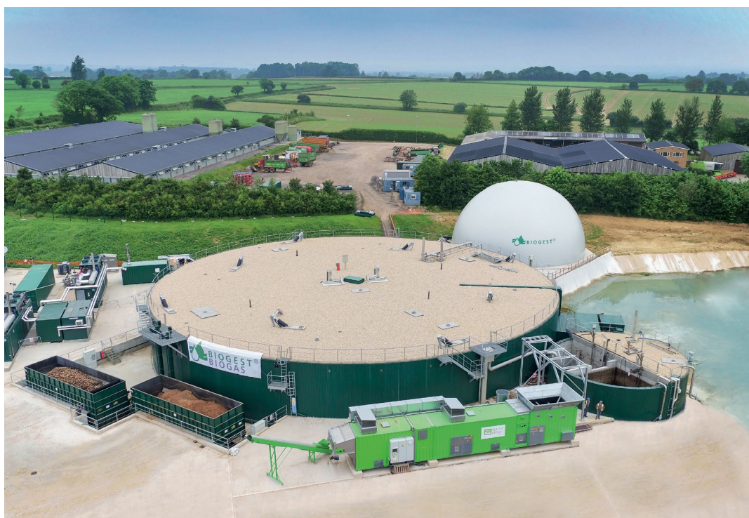
The facility will deploy Biogest's proprietary PowerRing
